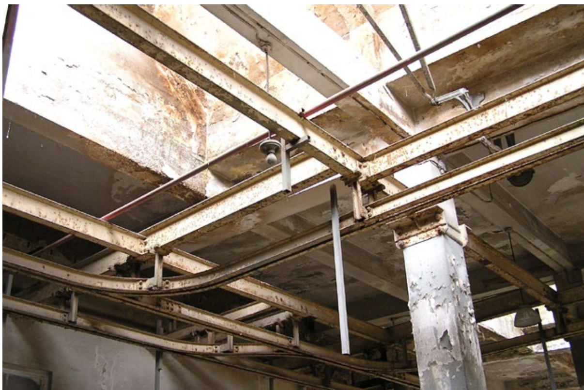
SLIKA 021 Interijer klaoničke hale: dio sustava za transport mesa, 2014. / IMAGE 021 Interior of slaughtering hall: part of the system for the transportation of meat, 2014
